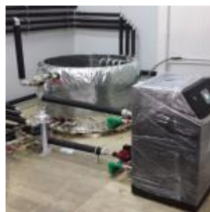
connection to thermal storage
